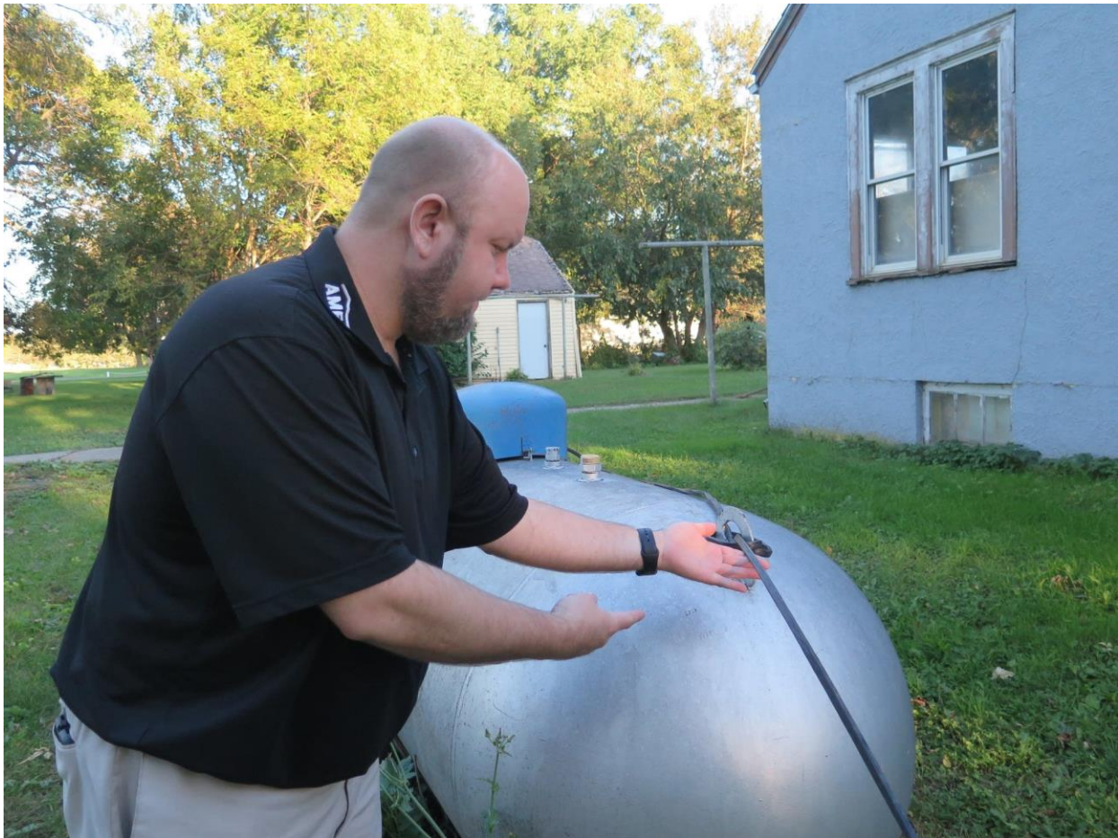
Ceylon City Council Member John Gibeau says Frontier Communications failed to complete this telephone line project. The cables have not been buried or attached to poles. This one crosses a propane gas tank. Mark Steil | MPR News
